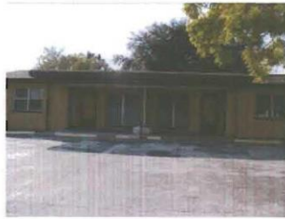
Area 7 – Residential Deterioration
