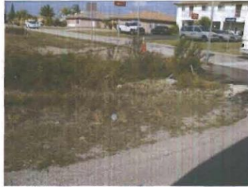
Area 9 – Neglected Infrastructure
