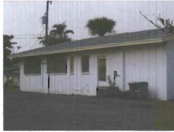
Area 6 – Residential Deterioration
